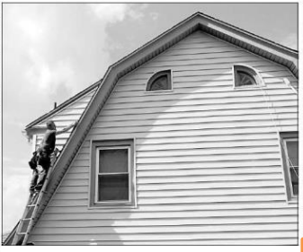
Roofer Hernan Jimenez balances on his ladder to fix a roof in Abington. CLEM MURRAY / Staff Photographer
